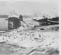
NOW YOU DON'T — What looks like the results from a direct hit from a buzz bomb is the old Plant Dispensary after riggers began wrecking it. The medical facility was built in 1936.
